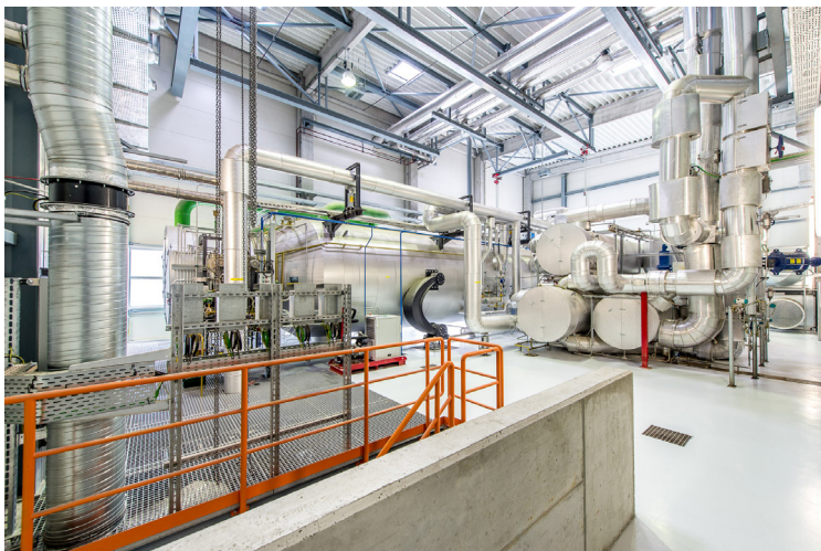
Turboden 5 MW ORC unit in CRH cement factory in Slovakia.
