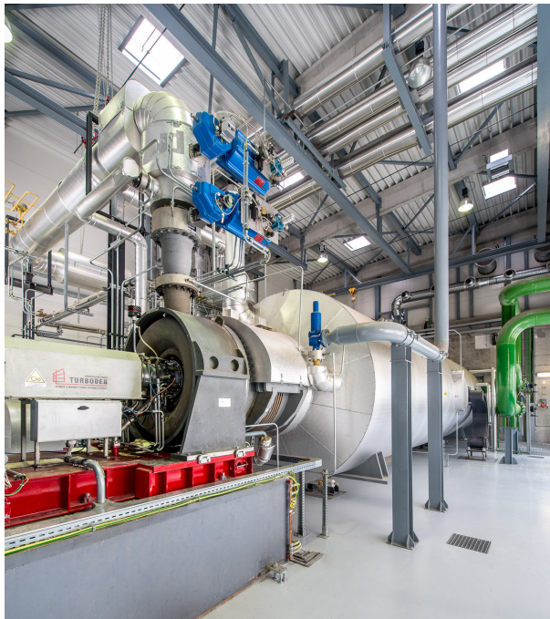
Turboden 5 MW ORC unit in a CRH cement factory in Slovakia.
